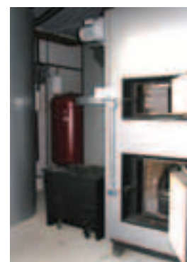
Fig. 3 320kW Biomass boiler at HDC.
