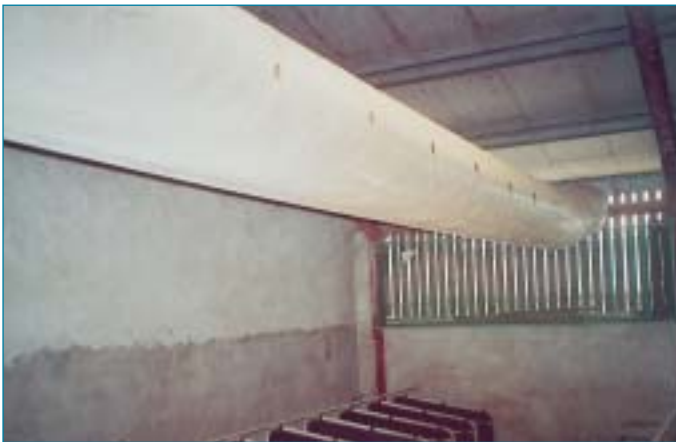
Polythene duct air distribution system
