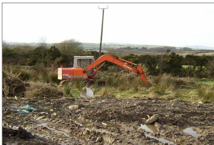
Fig 10: Damage to wetland is not permitted
